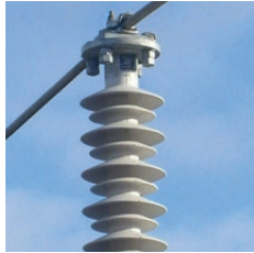
Negative feeder fixed to masthead
